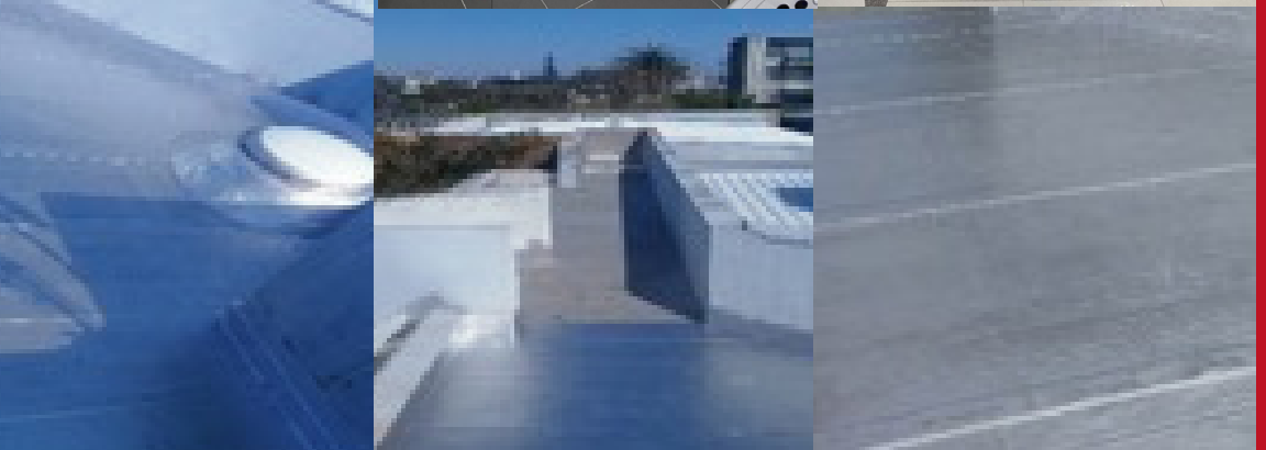
South African Bureau of Standards (SABS) Office building Waterproofing a section of the roof above main Entrance Sub Contractor for Cuecon Project Location: Mowbray Cape Town
