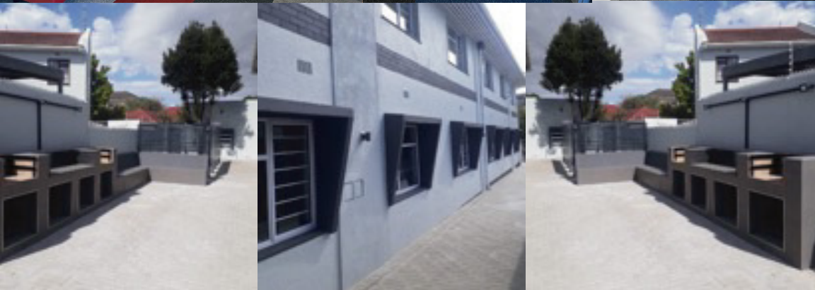
Removing of existing soft and hardscapes interior and exterior painting and waterproofing Location: Plumstead
