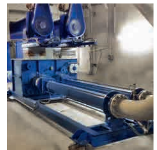
Conveyance of dewatered sewage sludge: KL80RQ110.4+110.4 Progressing cavity pump
