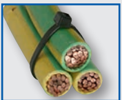
Nylon Cable Tie Tensioned/Cut/No sharp edges
