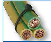
Nylon Cable Tie Tensioned/Cut/No sharp edges
