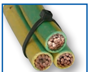
Nylon Cable Tie Tensioned/Cut/No sharp edges
