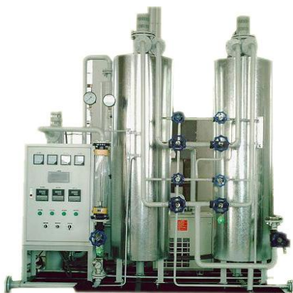
C. Hydrogen Generating Plant by Ammonia Decomposition
