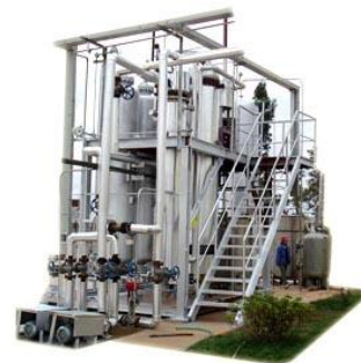
B. Hydrogen Generating Plant by Methanol
