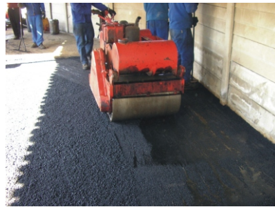
Compaction using a steel-wheeled pedestrian roller. Note handwork next to the wall
