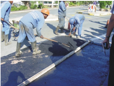
Using a lute (the flat side of rake) to spread hot mix. Note the levelling bar a
