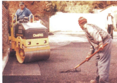
After initial compaction, a rakeman spreads premix to fill low spots ahead of the second (half-width) roller pass
