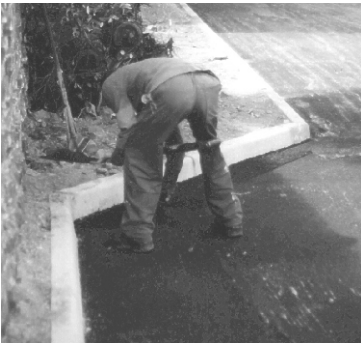
A skilled hand finisher ensuring that tight corners and kerb areas are neatly finished
