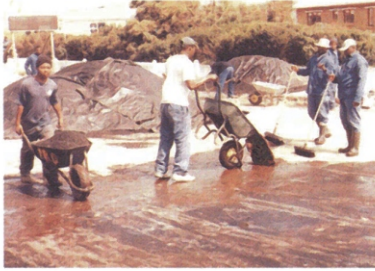
Brooming prime over the granular base while premix from covered stockpiles is barrowed to the worksite
