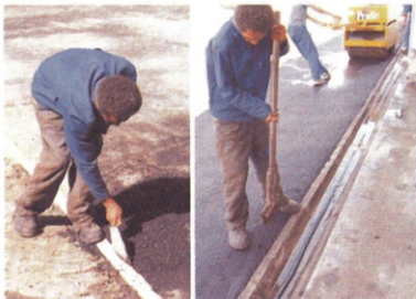
Handwork: cleaning up the edge with a trowel (left) and hand stamping. Note the neat edge to the concrete
