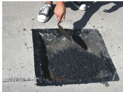
A pothole prepared for patching. Note the neatly cut edges sloped at an angle to receive new hot mix
