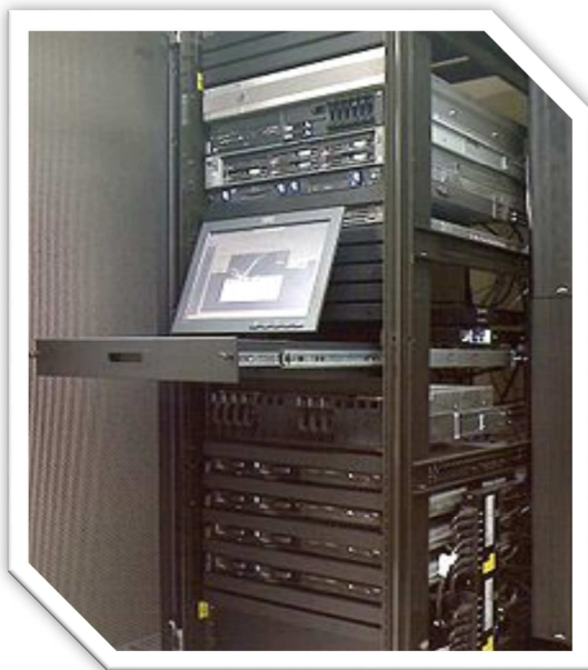
A Server rack in a Data Centre connected to a KVM Switch
