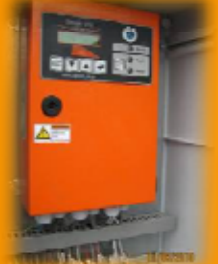
Control Unit Inside Protection Enclosure
