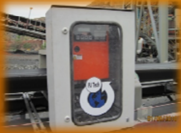
Control Unit in Protection Enclosure
